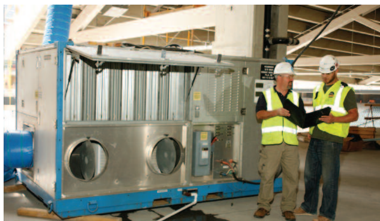
Polygon technician Joe Schmitz (left) and Eric Keleny from M. A. Mortenson Co. check the performance of the Polygon humidity control unit.
