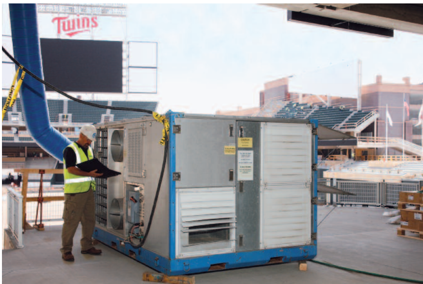
Temperature and relative humidity readings are collected by Polygon operations technician to determine performance of the HCU-6000.
