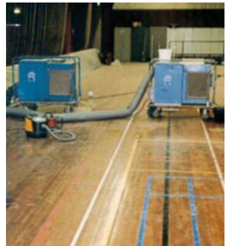
Dehumidification of sports floor.
