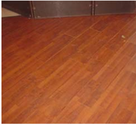
Damaged laminated floor.
